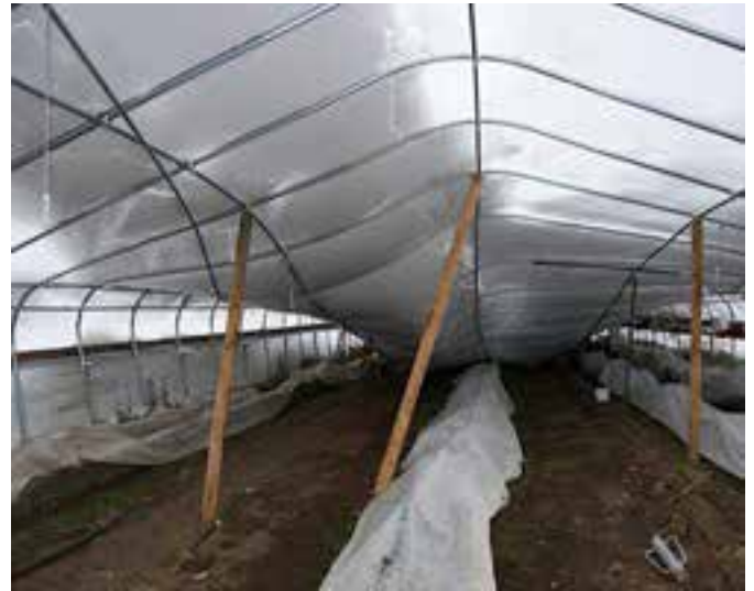
Snow load collapsing a greenhouse. Credit Cornell Vegetable Program
