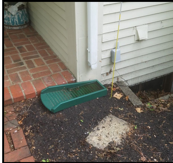
Figure 3.16: Water downspouts are directed at splash blocks angled toward the house instead of away
