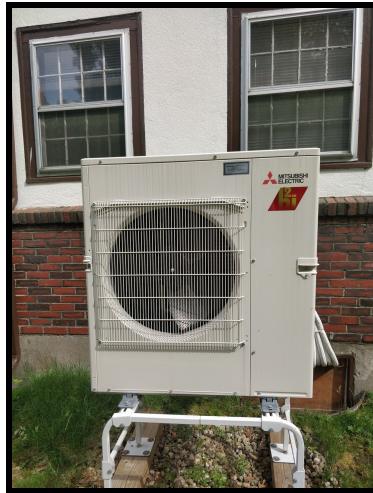
Figure 4.8: Air-Source Heat Pump outside Miller Hall.
