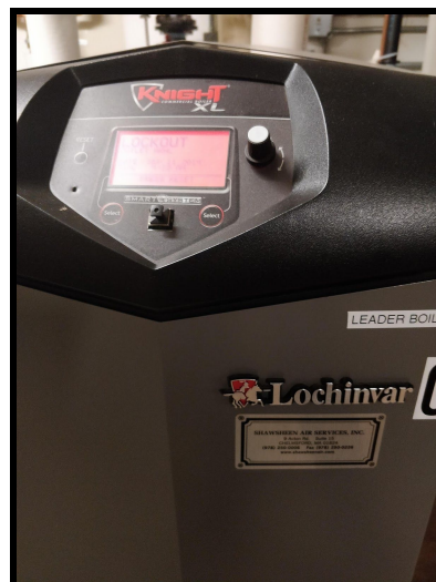
Figure 4.10: New Lochinvar Boiler in Malloy
