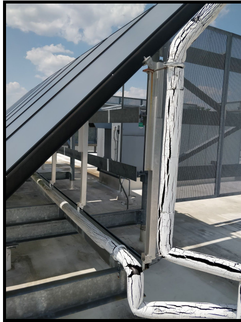
Figure 4.15: New Hall solar thermal system and damage
