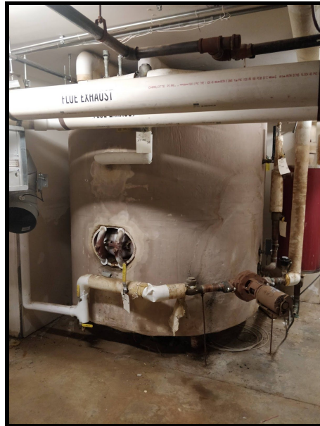
Figure 4.9: Malloy Water heater in need of replacement
