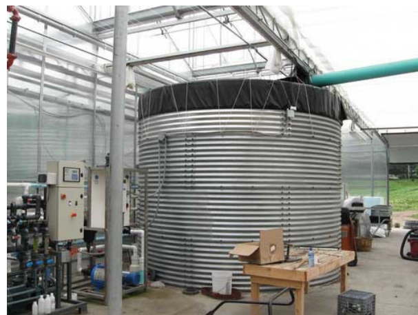
Rainwater Holding Tank
