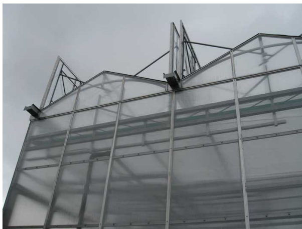
Rainwater Collection System
