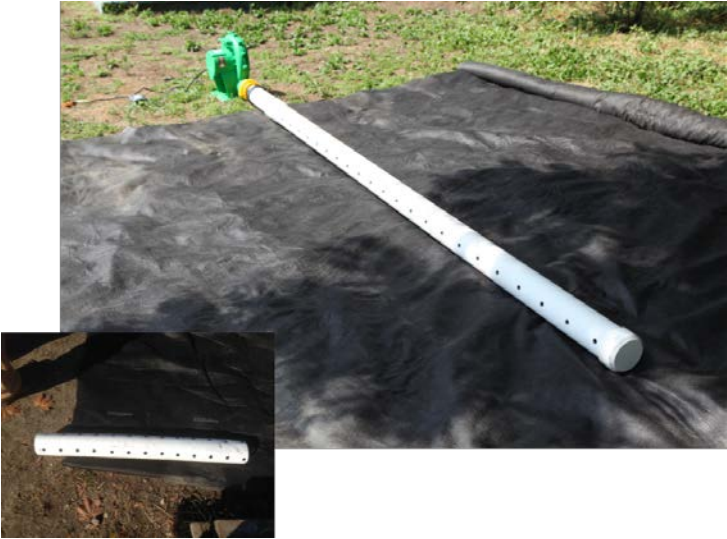
Figure 5. Connected PVC pipe with blower
