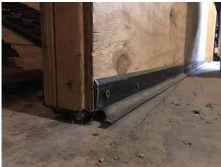
Worn out door seals can be a place for major air leakage. Be sure to inspect and replaced door sweeps and weather striping when necessary.
