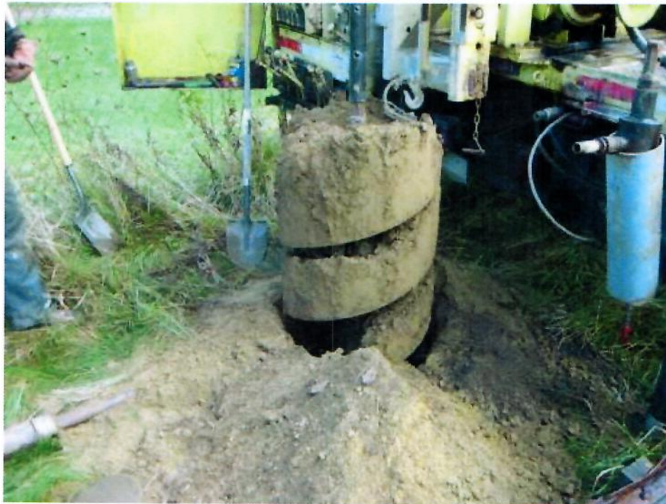
Figure 7. Excavating a Hole for a Drilled Pier Using a Truck-Mounted Drilling Rig.
