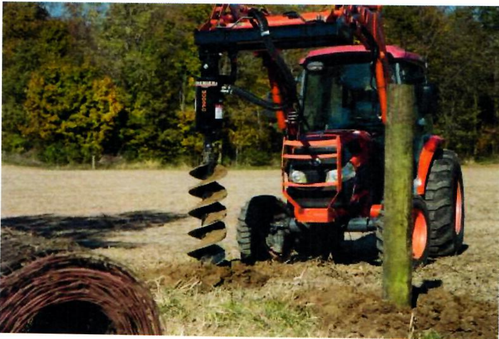
Figure 16. Drilling a Concrete Pier Hole Using an Auger Mounted on a Tractor.
