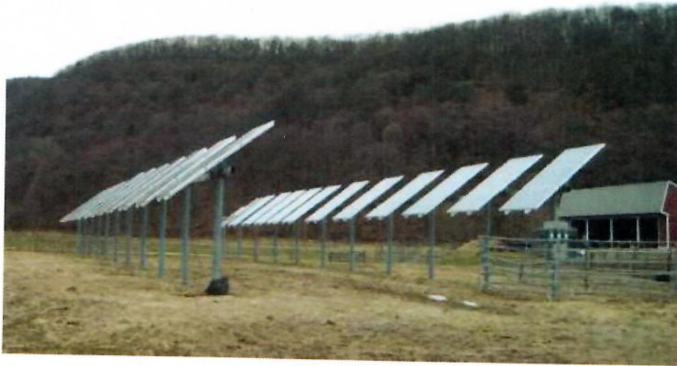
Figure 3. Typical Elevated Ground-Mount PV Solar Panel Array. (UMass Agricultural Farm – S. Deerfield, Ma.)
