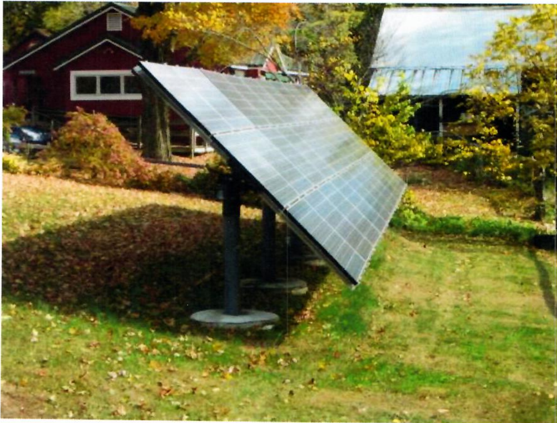
Figure 10. Drilled Concrete Pier Supported PV System - Sunderland, Ma.
