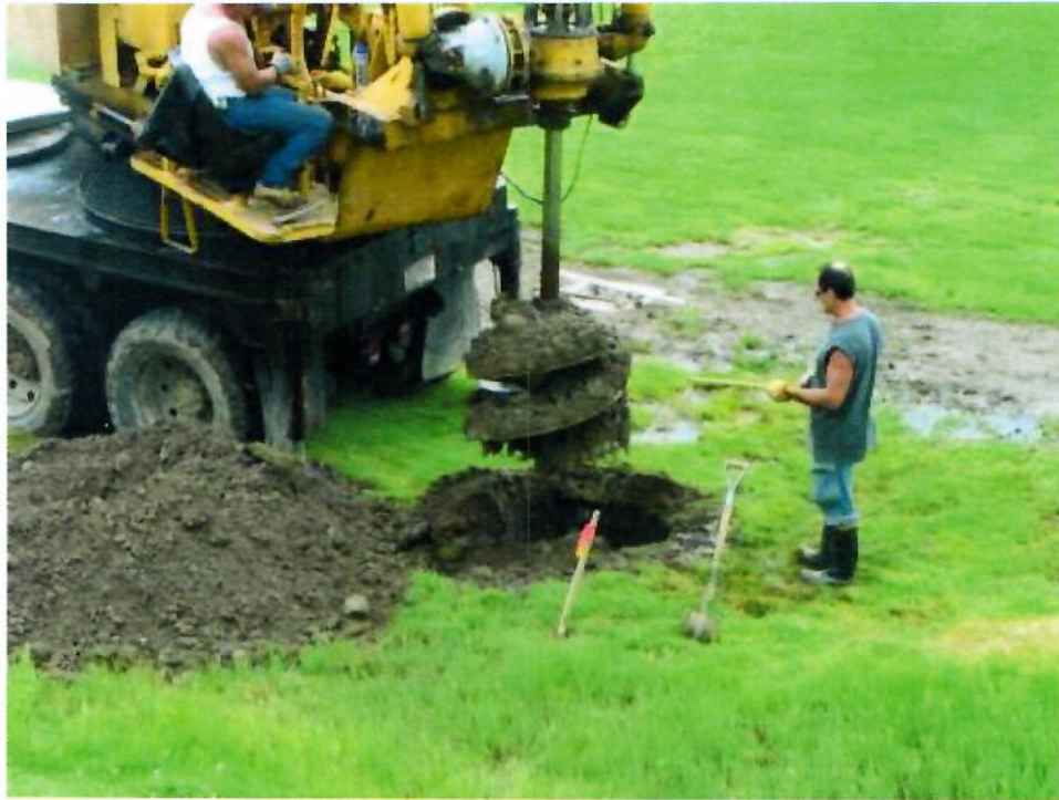
Figure 6. Excavating a Hole for a Drilled Pier Using a Truck-Mounted Drilling Rig.
