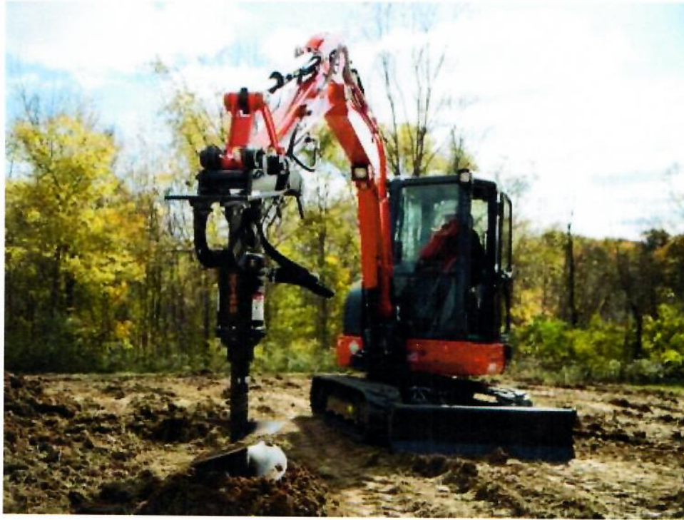
Figure 18. Drilling a Concrete Pier Hole Using an Auger Mounted on a Compact Excavator.
