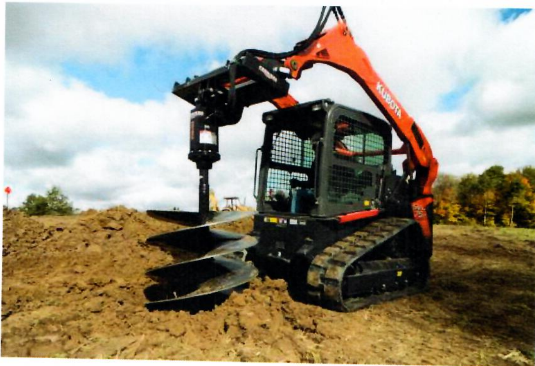
Figure 17. Drilling a Concrete Pier Hole Using an Auger Mounted on a Skid Steer.
