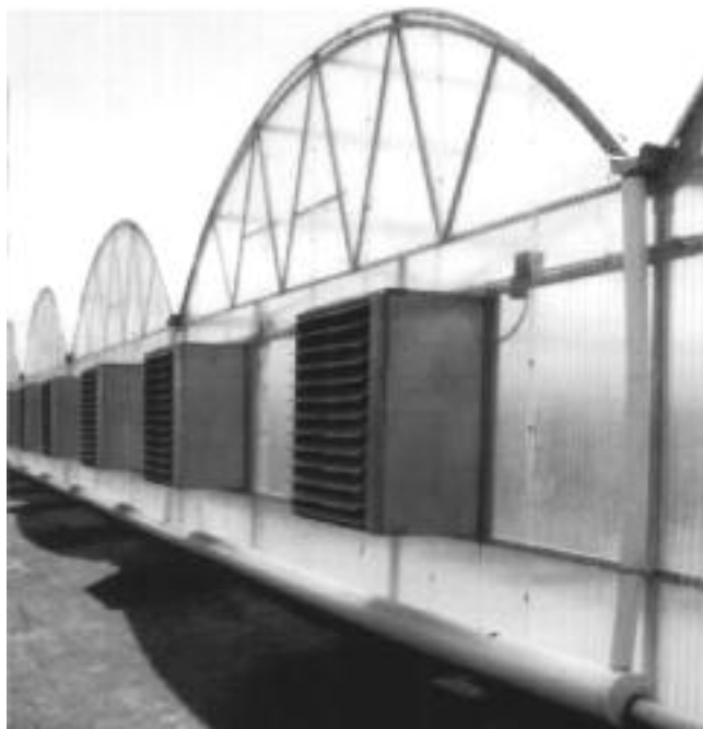
Exhaust fans are essential to remove heat even in the winter.
